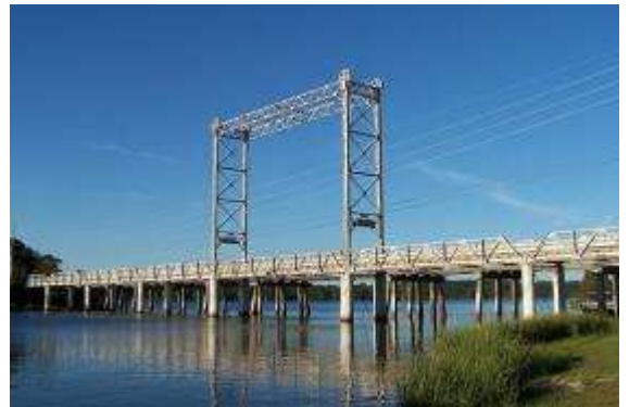
In 1914, the Caddo Lake Drawbridge replaced a ferry that transported people across Caddo Lake at Mooringsport.
